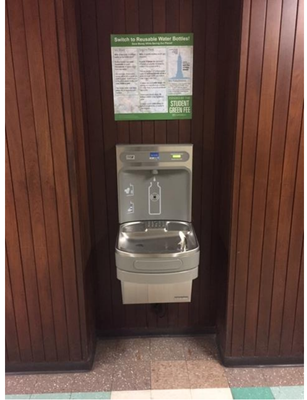
New Elkay refillable water station
