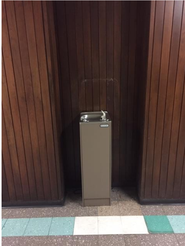
Original water fountain
